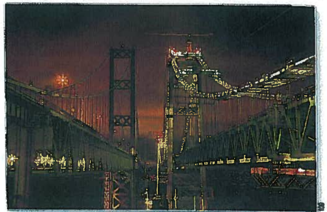
Figure B.2.1-1. Tacoma Narrows Bridge, WA. This Bechtel-Kiewit joint venture was completed within budget, on schedule, and with an exemplary safety record, despite high winds and strong deep-water currents and tides.
